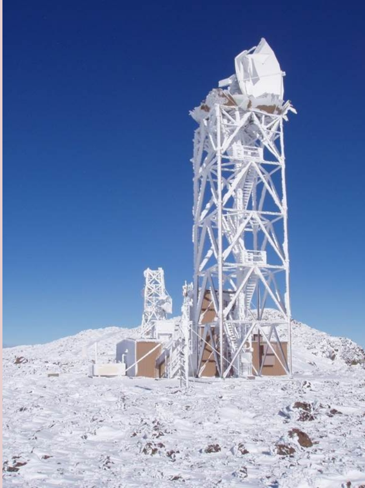
Figure 4-4 NWS Reno Radar Damage from Wind (December 2008)
