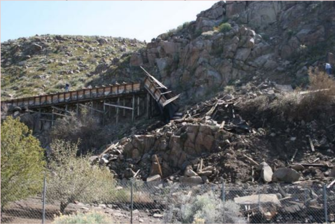
Rock fall damage to water flume
