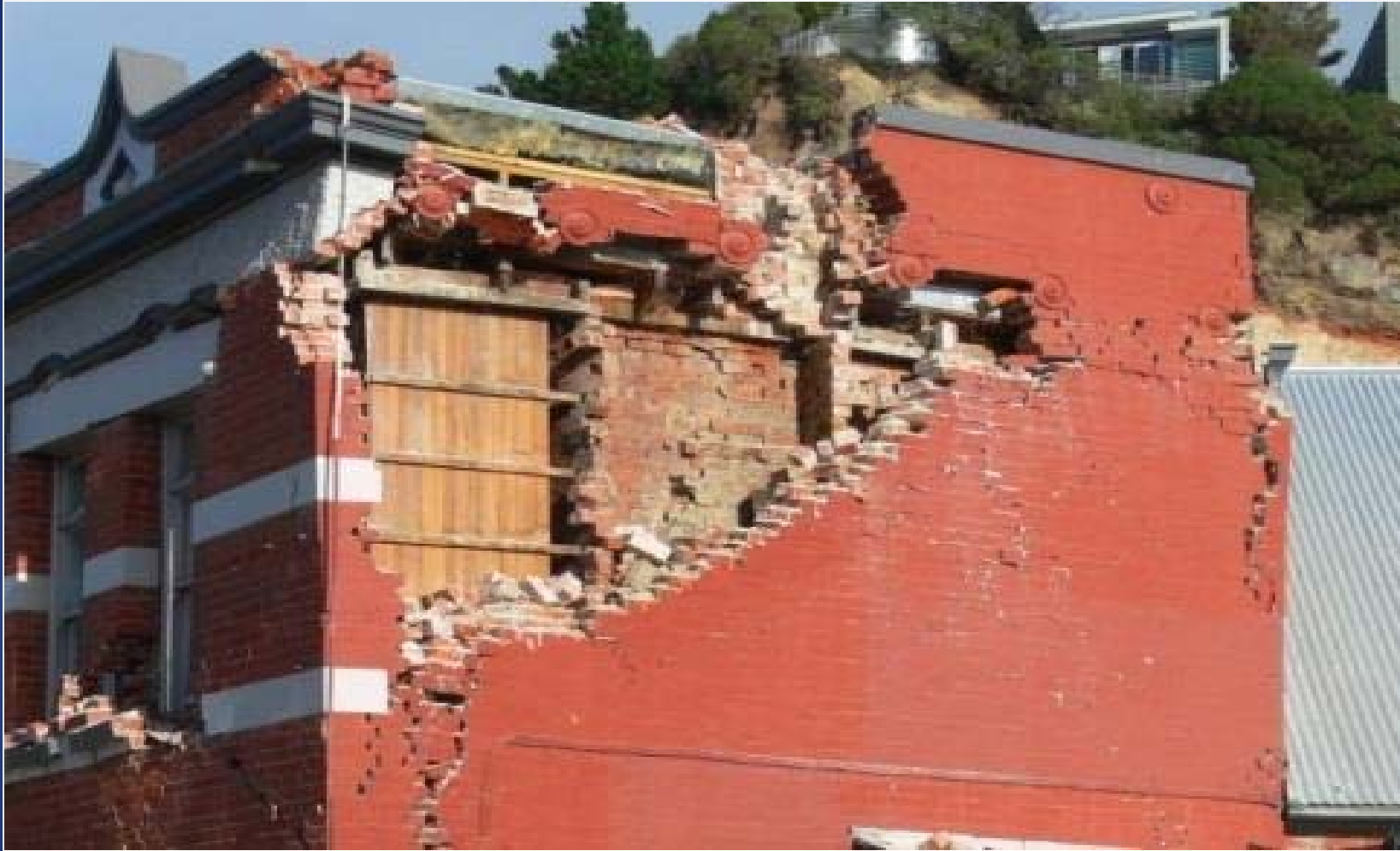
June 13, 2011 Magnitude 5.5 and 6.0 earthquakes 3 mi (5 km) away
